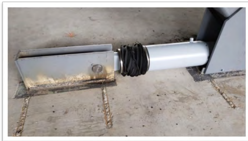
Viscous dampers are built into the steel and concrete structure of the building.
